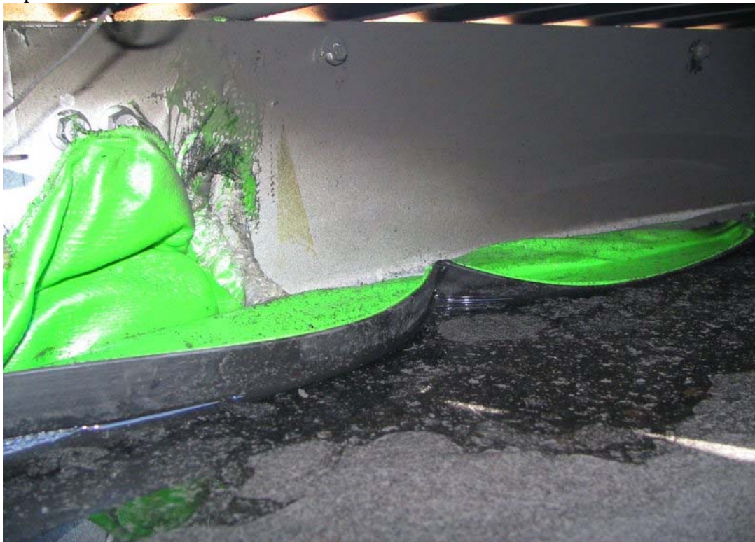
Figure C63 Damage to bladder tank liner resulting from pre-radiation and flame exposure.
