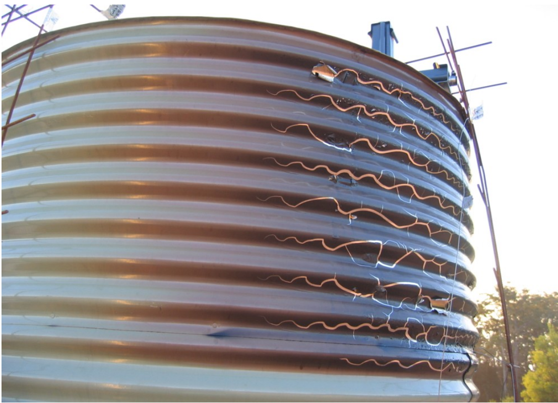
Figure C19 Tank five surface scorching above water line.
