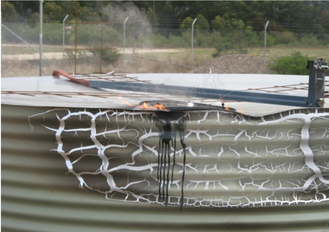
Figure C4 Tank one slight structural damage due to flame exposure
