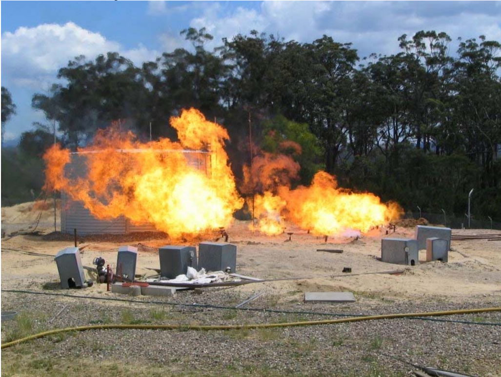
Figure C60 Bladder tank pre-radiation and flame exposure.
