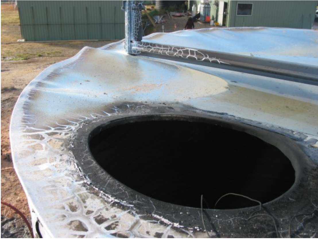
Figure C40 Tank 7 damage resulting from structural exposure.
