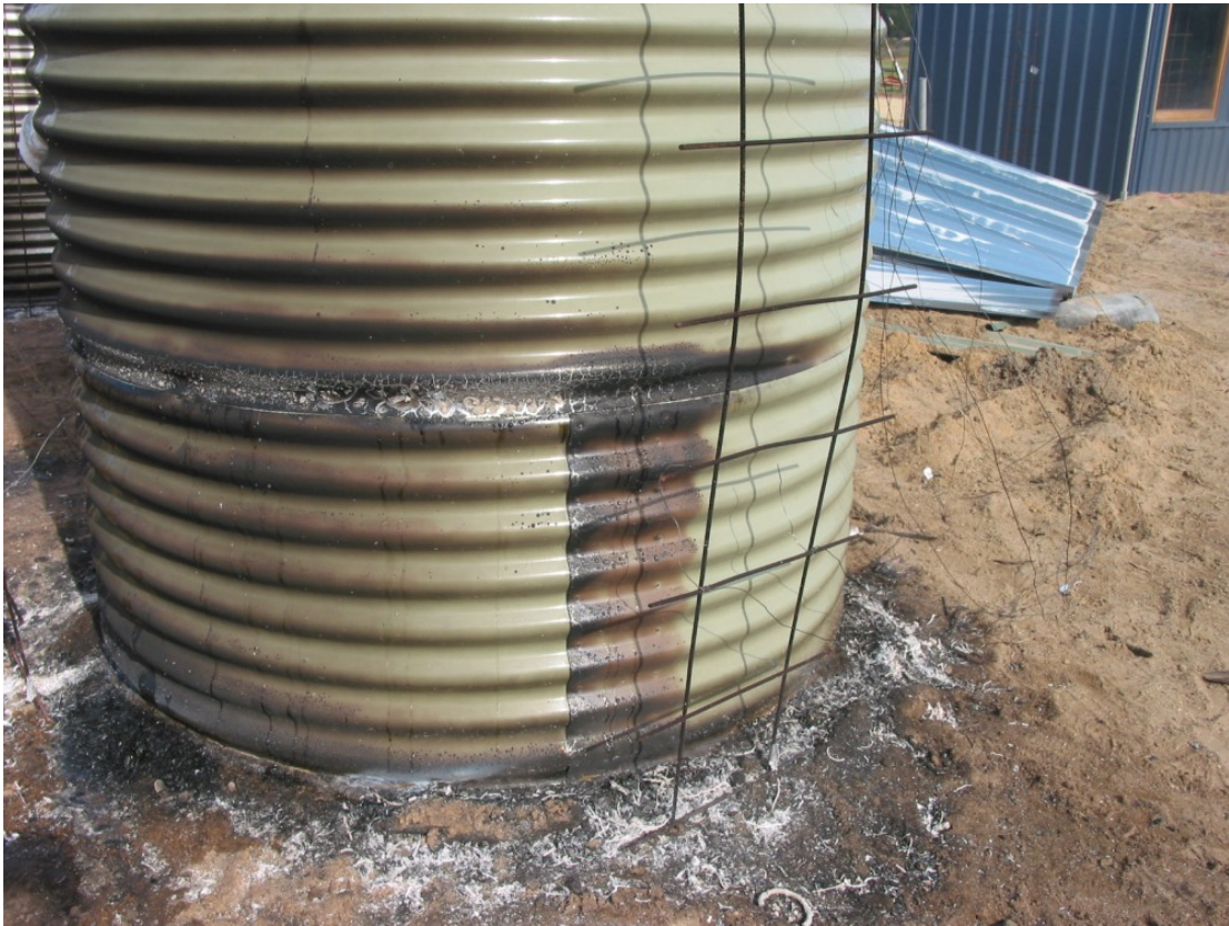
Figure C22 Tank three water leaking from damage seams.
