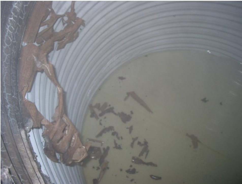
Figure 16 Internal polymeric coating damage above water level
