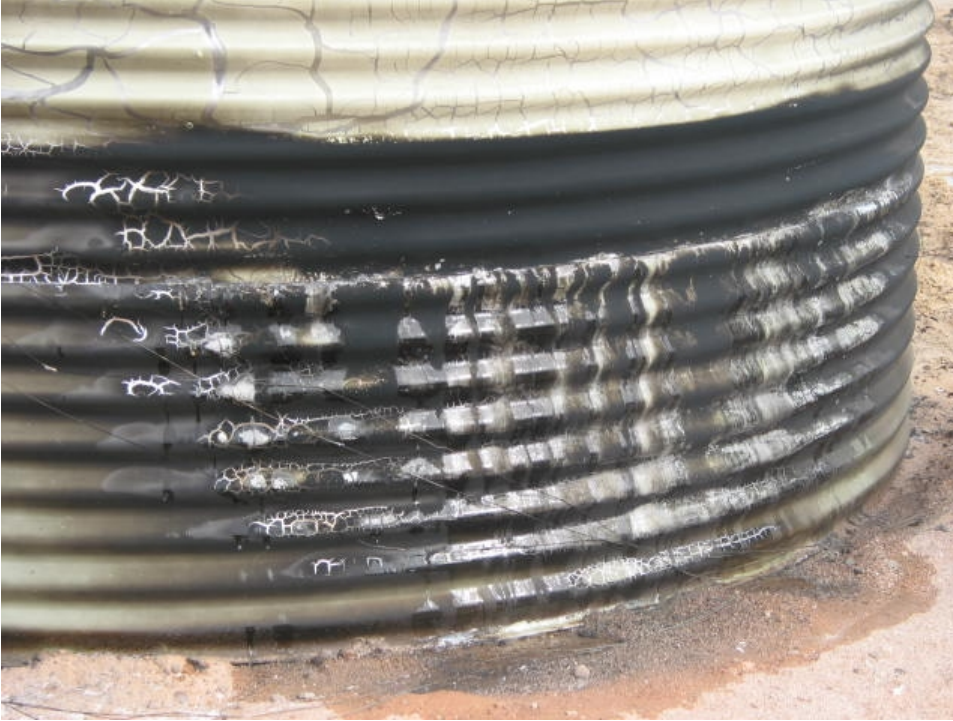
Figure 7 Experiment 3 - Structure exposure on metal coated tank
