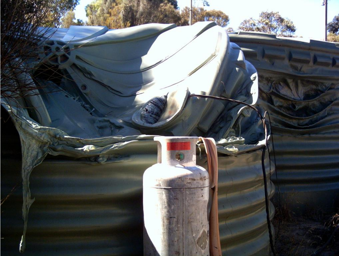
Figure 1 Example of water tank damaged, Eyre Peninsula
