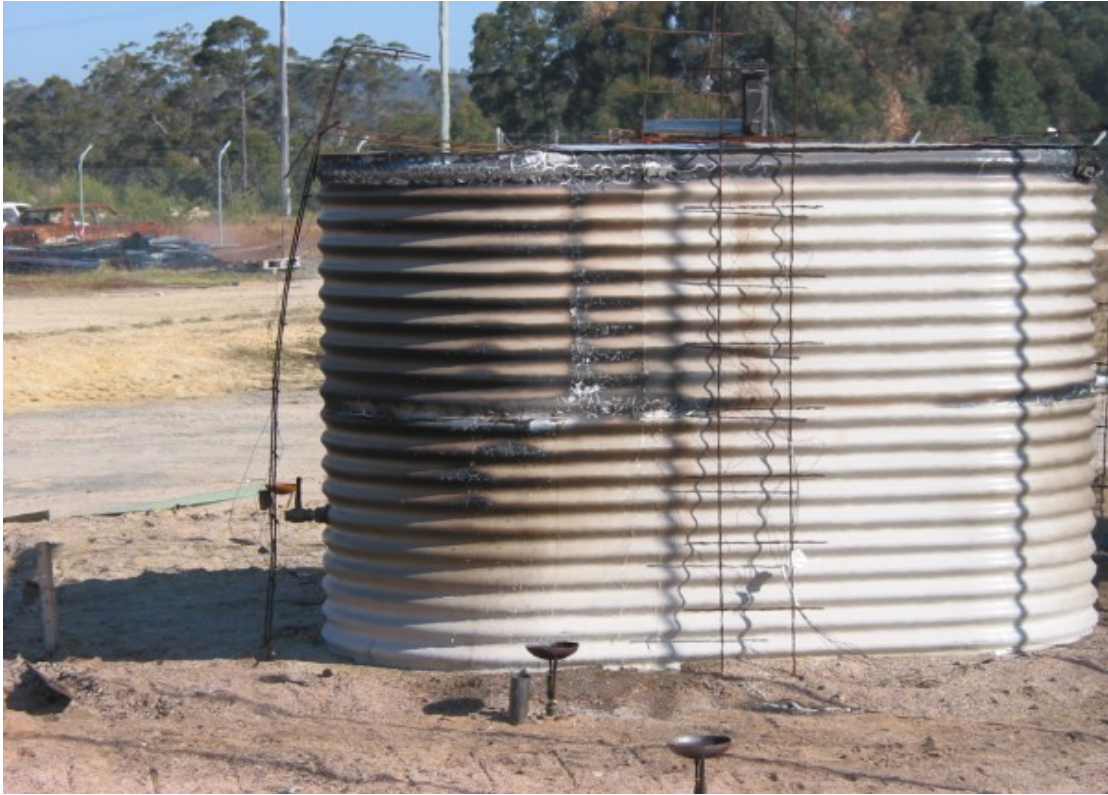
Figure C29 Tank two external damage due to flame exposure.
