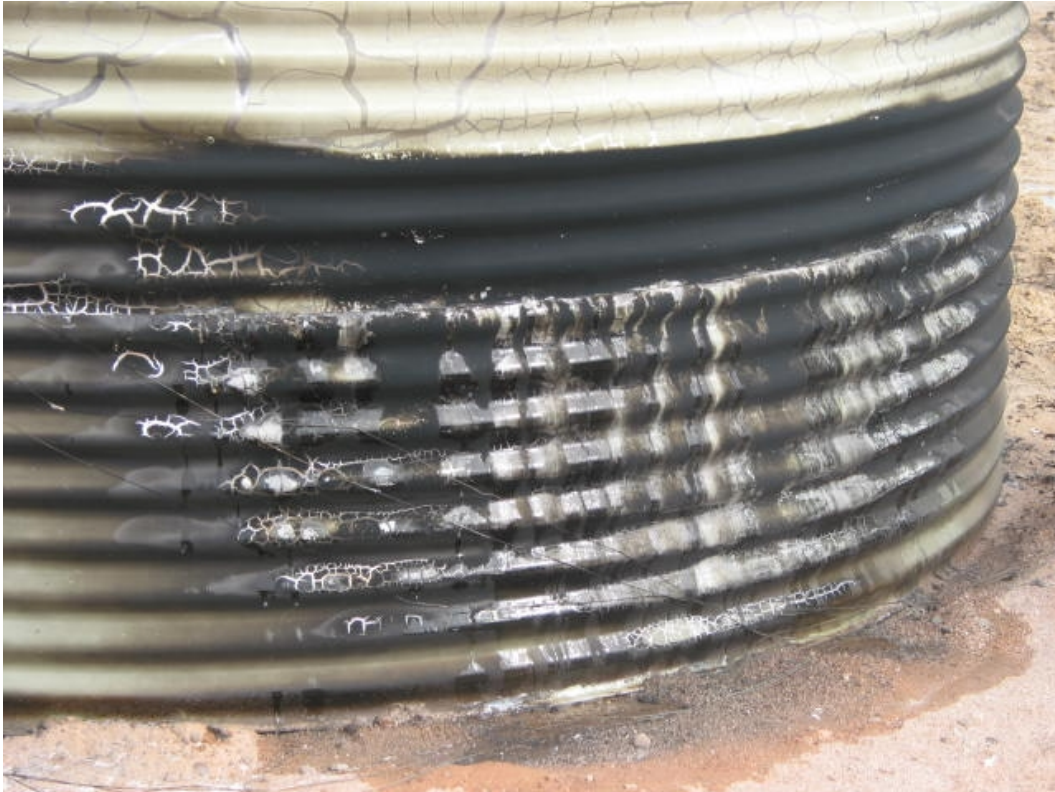
Figure C5 Tank one severe damaging resulting from structural exposure
