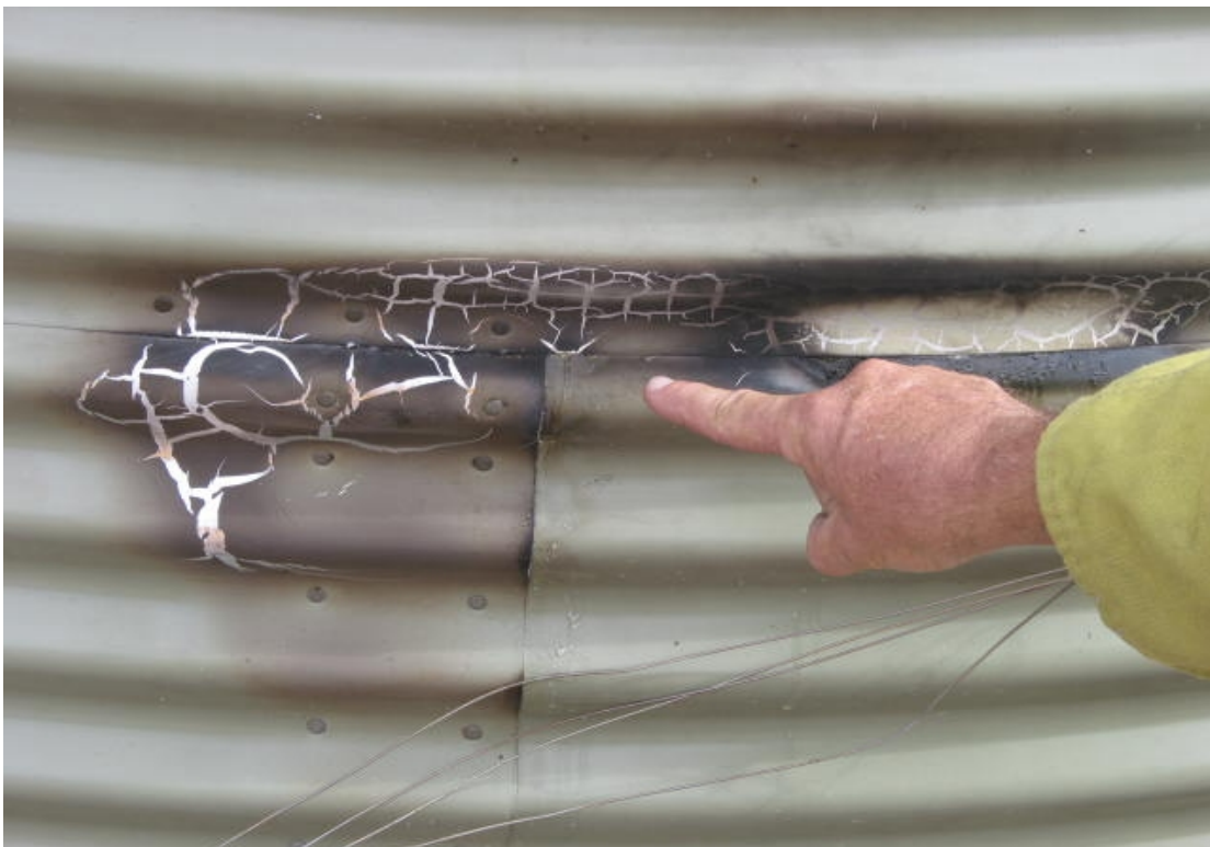
Figure C4 Tank slight damage to joints
