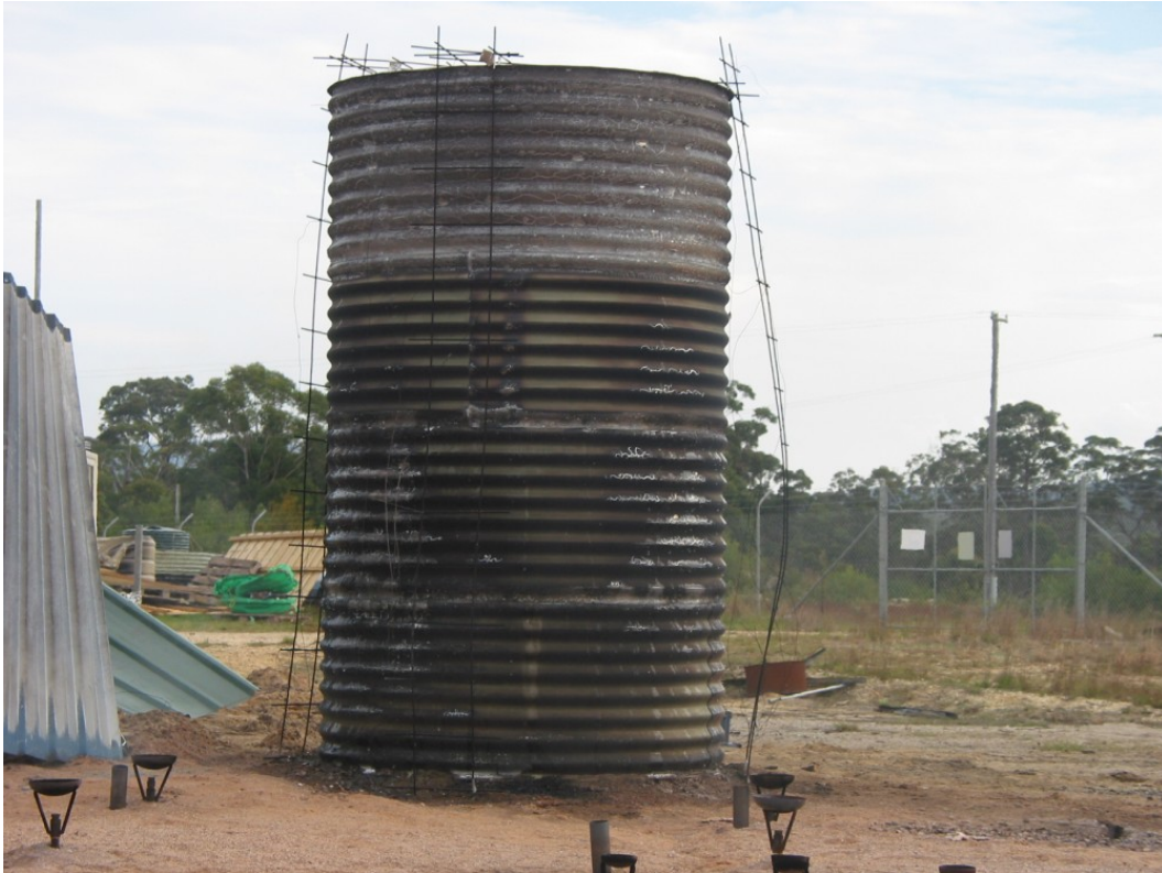
Figure C25 Tank three severe damage resulting from structural exposure.
