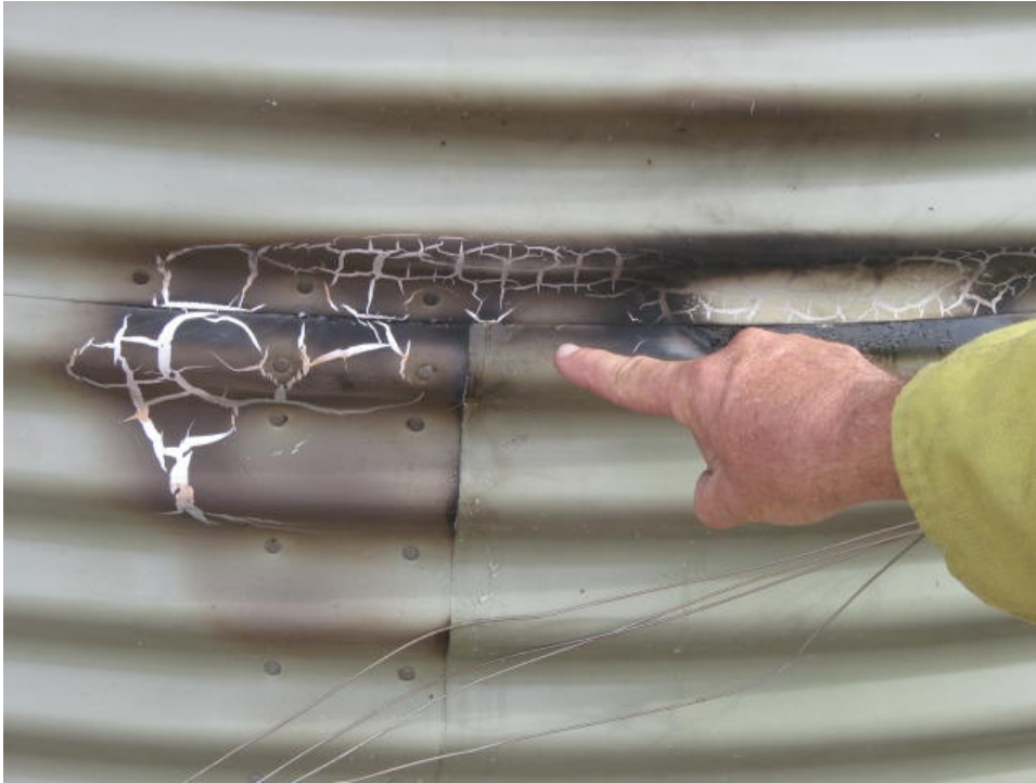
Figure 6 Experiment 2 - Leaf litter ignited and flame immersion exposure, small leaks from the seams
