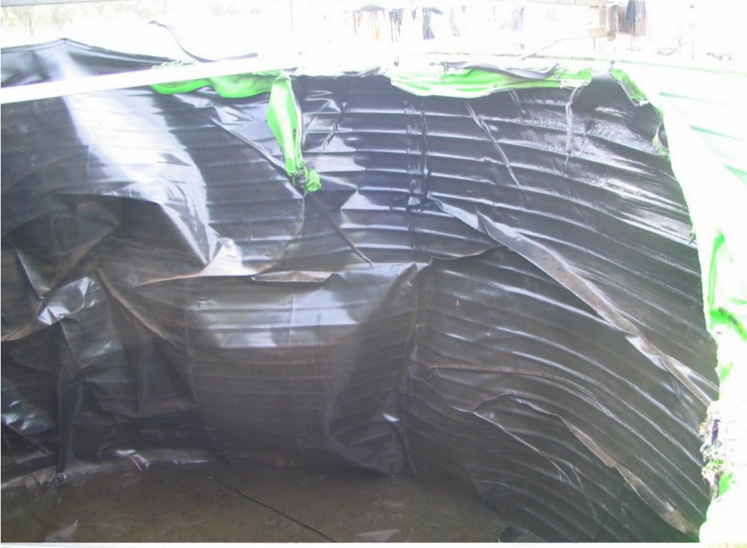
Figure C67 Damage to tank 9 liner resulting from structural fire exposure.
